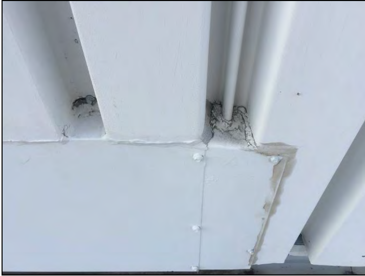
7. View of the non-asbestos grey caulking found on the exterior metal sidewalls of the penthouse mechanical room located on the top of the LBJ Building.
