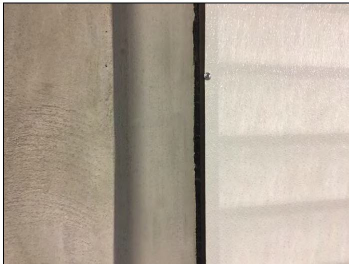
8. View of the non-asbestos stucco wall finish and the black caulking found around the plastic/fiberglass panels used to cover the old vents located within the SE stairwell.
