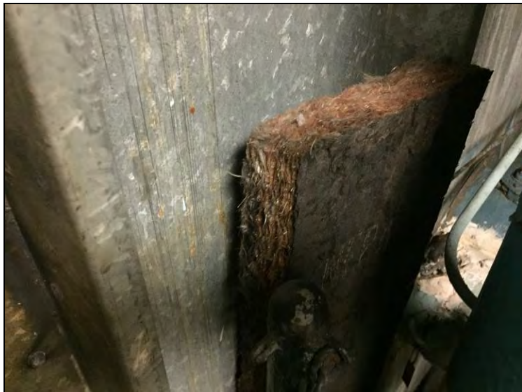
17. View of the non-asbestos black rigid insulation board found on the interior of the HVAC air handlers.
