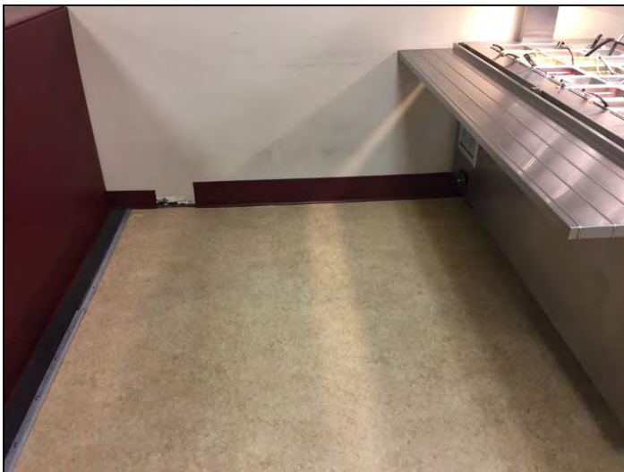
15. View of the non-asbestos gold sheet vinyl flooring found in the basement canteen.
