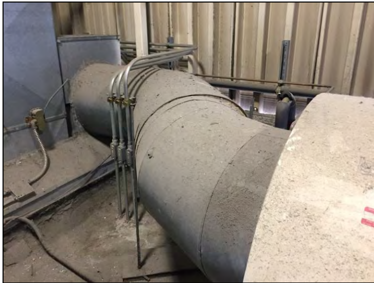
5. View of the non-asbestos dust found on the HVAC ducting and air handling equipment located in the penthouse.
