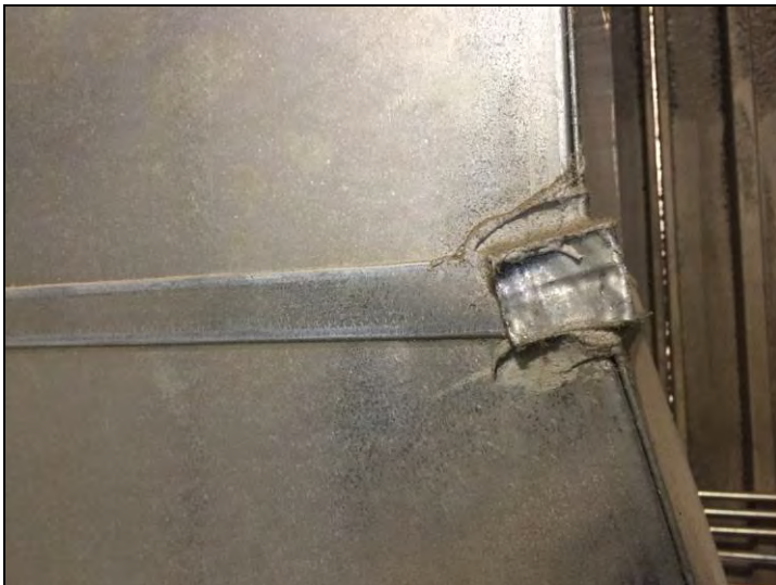
6. View of the non-asbestos grey caulking found on the exterior of the ducting and the air handlers located in the penthouse mechanical room.
