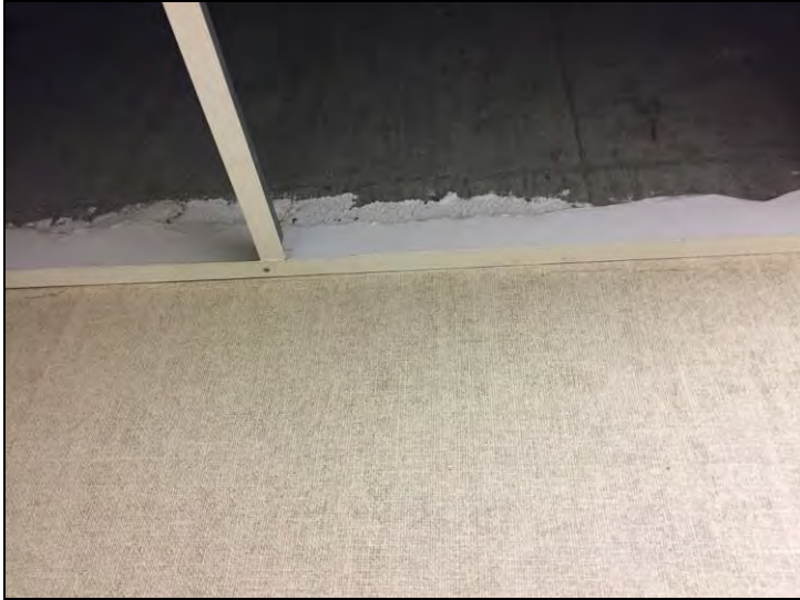
10. View of the non-asbestos plaster finish and vinyl covering found on the plaster and sheetrock walls found in various locations throughout LBJ Building.
