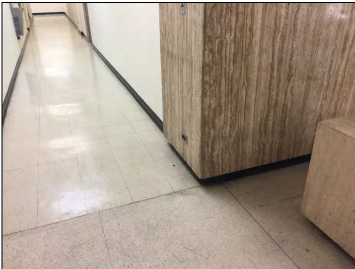
12. View of the new non-asbestos terrazzo flooring and travertine stone wall finish found in main elevator lobby area.
