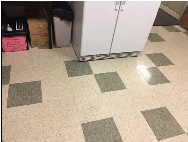
14. View of the new non-asbestos tan and grey vinyl floor tile found in the 2 nd floor breakroom.
