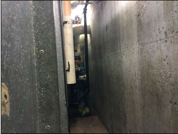
16. View of the non-asbestos TSI fiberglass pipe-run insulation found on the steam, chilled, roof drain and domestic water lines and exhaust from the emergency generator.
