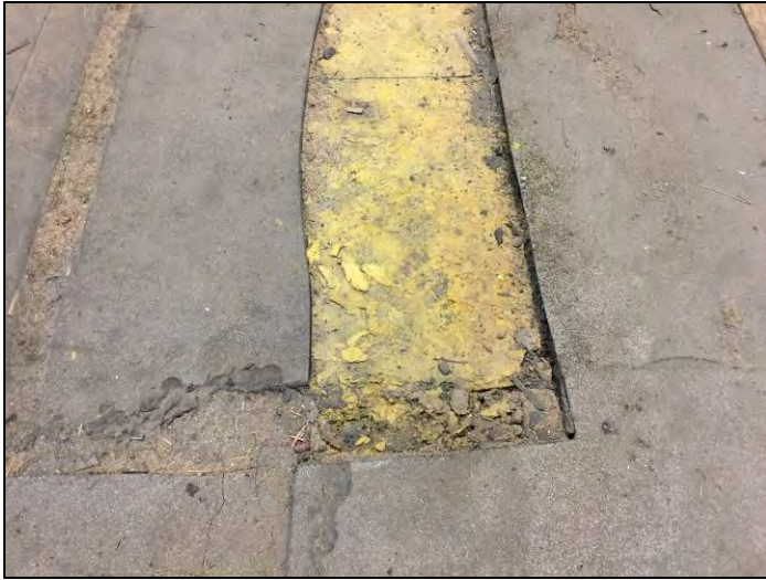
4. View of the non-asbestos yellow rigid fiberglass board found beneath the old asphalt roofing located in the penthouse mechanical room.
