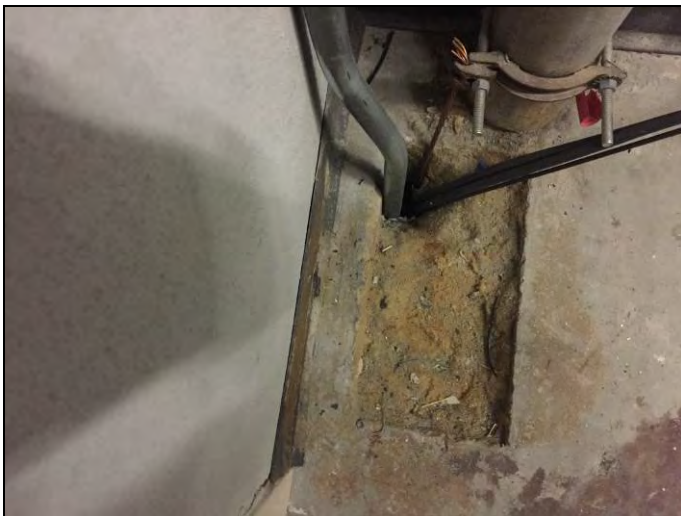
18. View of the non-asbestos foam insulation applied to the pipes and conduits at penetrations through the concrete floors.
