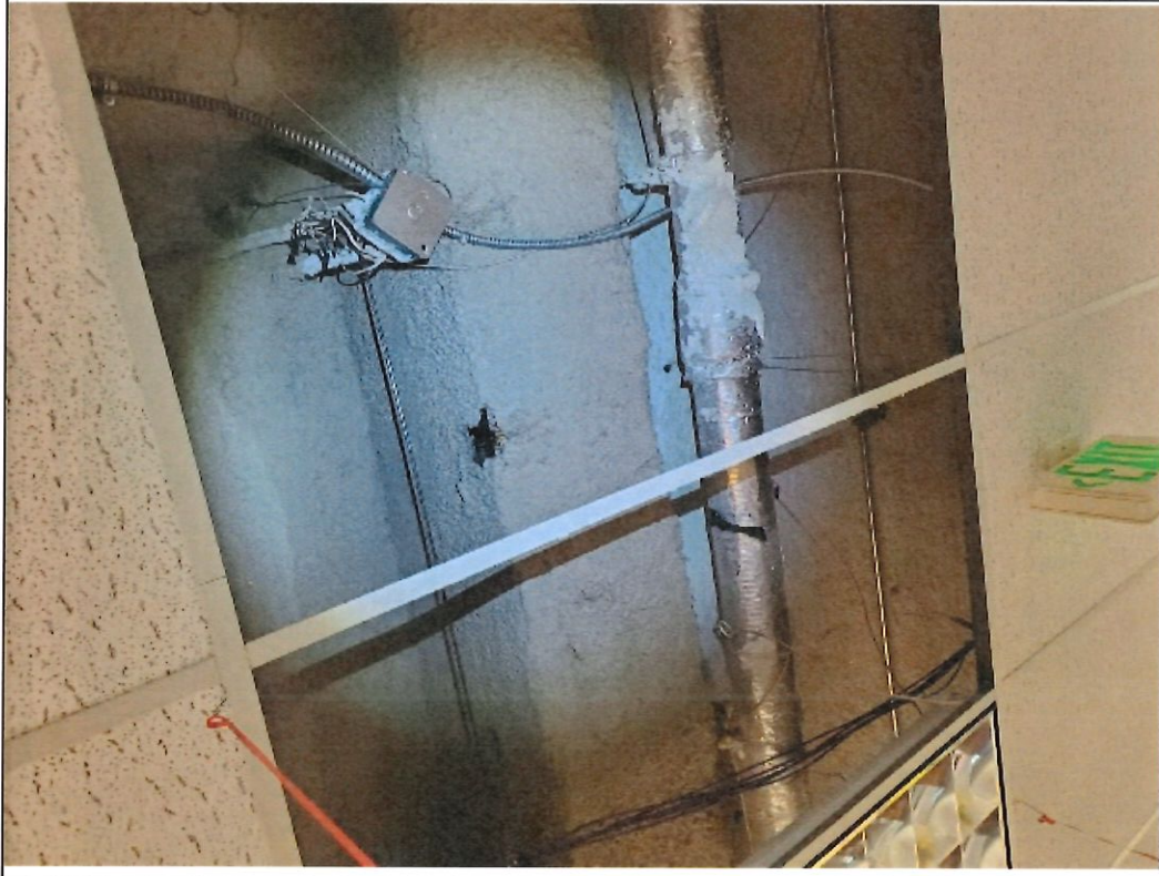
7) Saturated spray-on fireproofing within ceiling cavity. Exposed metal wiring visible where fireproofing material was no longer present.
