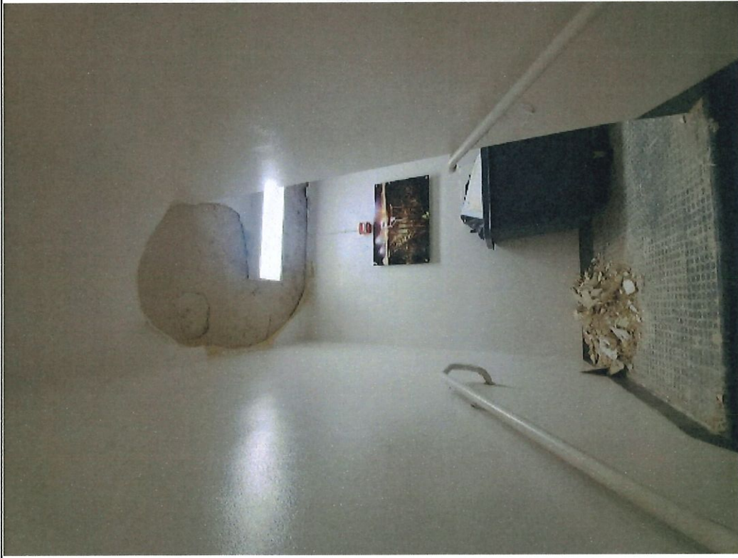
5) Water-damaged plaster material on the ceiling within the main stairwell.
