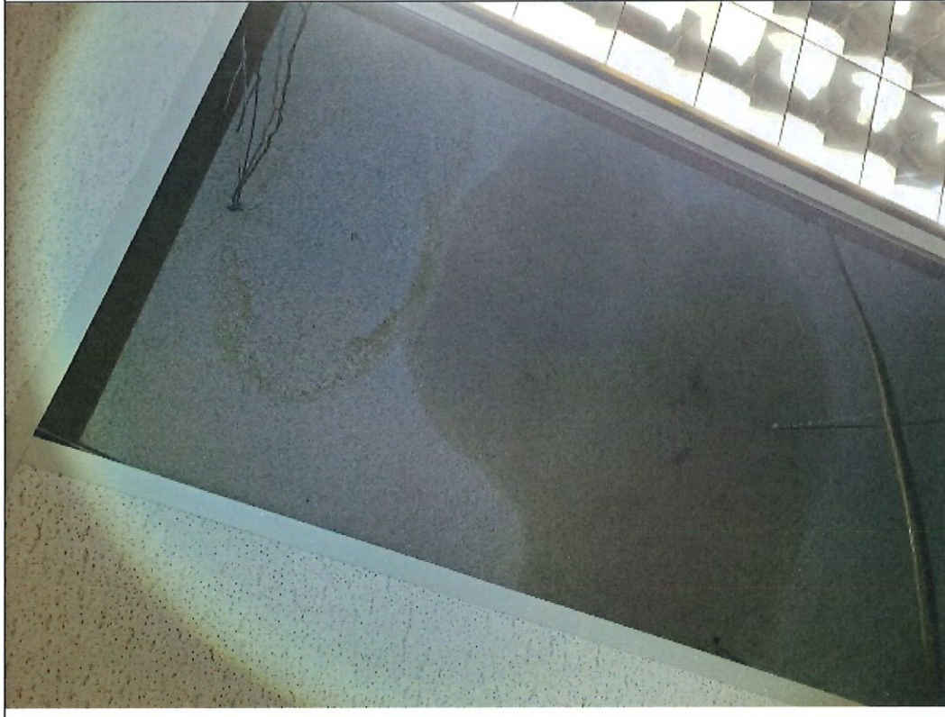
1) Spray-on fireproofing material actively wet adjacent to previously saturated material within a ceiling cavity.
