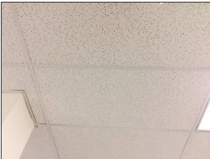
6. View of the non-asbestos 2'x4' suspended ceiling tiles found in various locations throughout the building.
