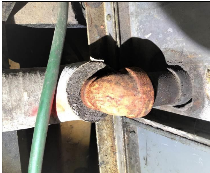
8. View of the canvas covering found over the asbestos felt paper on the black pumice-like pipe insulation. This material is found in various locations throughout the building.
