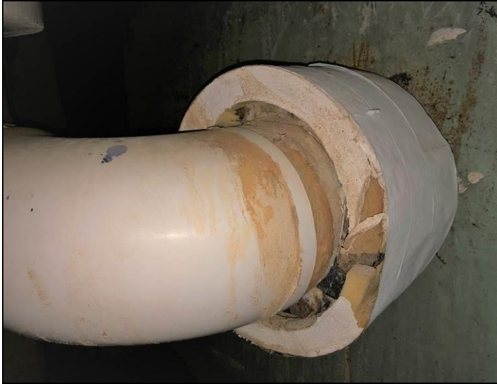
19. View of the non-asbestos TSI (new fiberglass) pipe-run insulation with white plastic fittings found in the basement mechanical room. Also shows the non-asbestos coating applied to the exposed end of the insulation.
