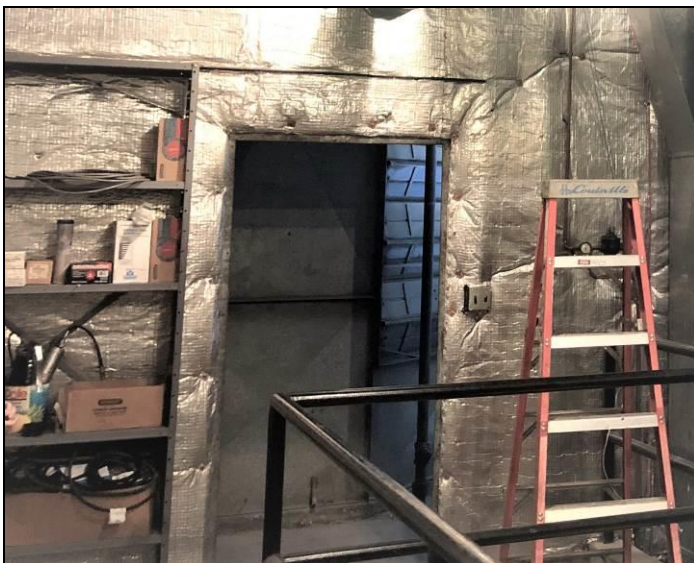
21. View of the non-asbestos foil covered fiberglass insulation found on the metal wall between the air handler and the penthouse mechanical room. Similar materials were found on the exterior of the HVAC ducts found in various locations throughout the building.
