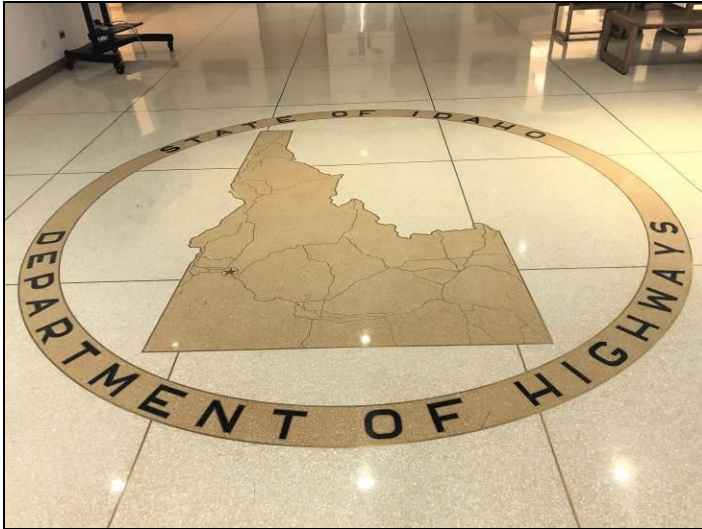
13. View of the non-asbestos terrazzo flooring located in the main entry lobby.
