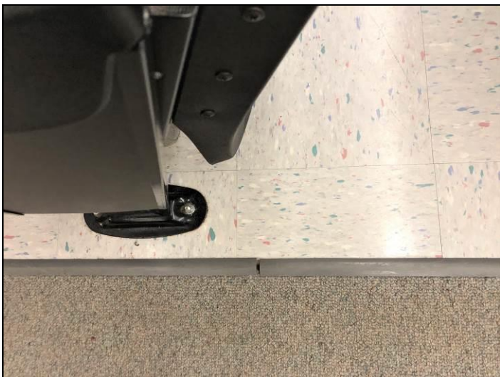
15. View of the new non-asbestos 12-inch vinyl floor tiles found within the auditorium located on the main level of the building.
