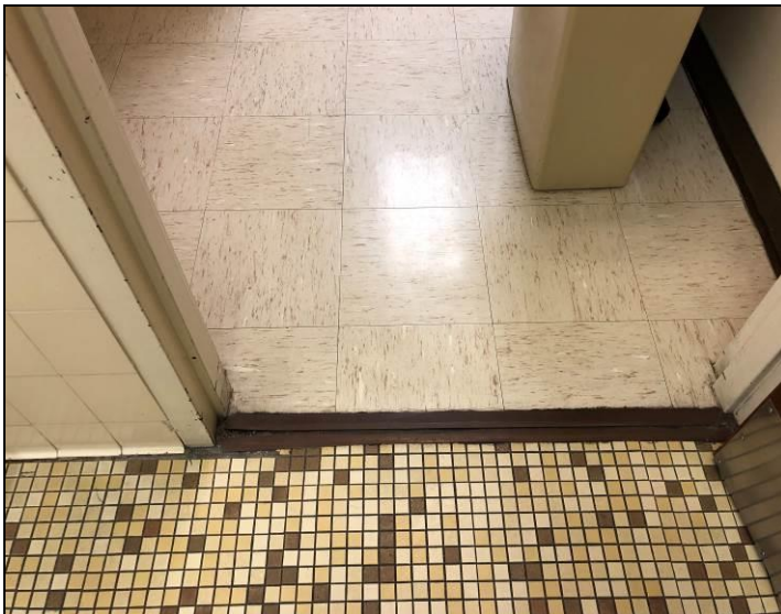
12. View of the non-asbestos ceramic grout found on the restroom walls and floors located throughout the building. Also shows the non-asbestos 12-inch floor tiles found in various locations.
