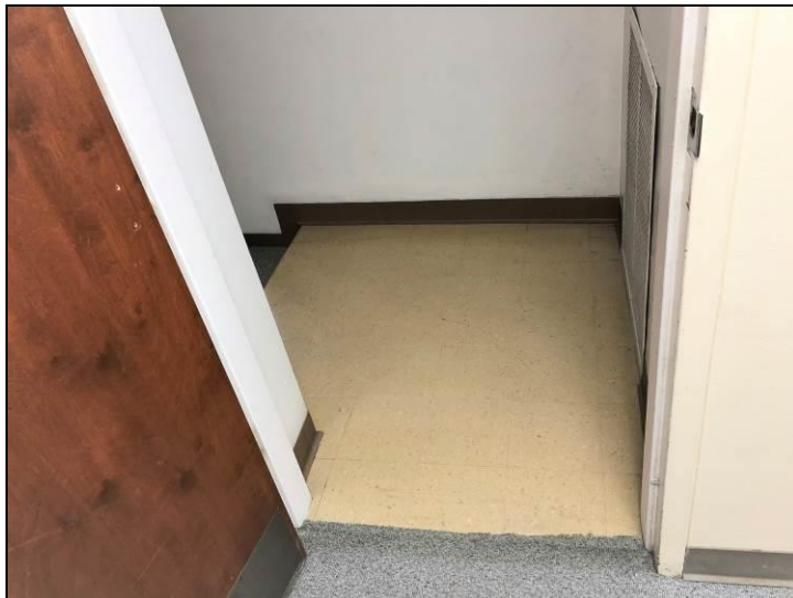
14. View of the non-asbestos 9-inch vinyl floor tile located on the 1 st floor. Dark brown, tan, and yellow mastic were used to adhere the tile to the concrete flooring. Similar tile is concealed beneath the blue raised dot vinyl flooring located in the stairwells.
