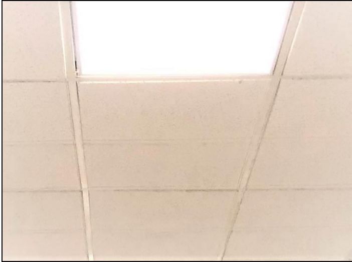
7. View of the non-asbestos 2'x4' (2'x2' pattern) ceiling tiles found in various locations within the building.
