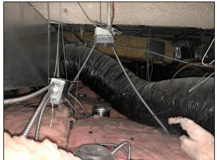
20. View of the non-asbestos poly covered and uncovered fiberglass duct insulation. Also shows the non-asbestos batt insulation found above the ceilings.
