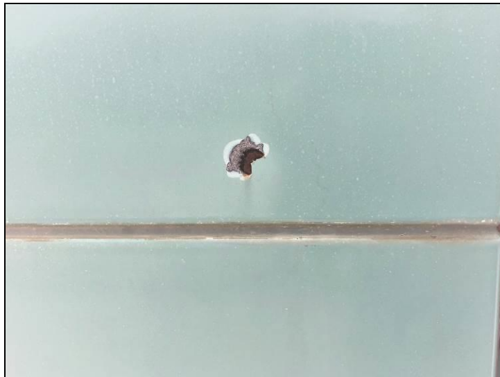
2. View of the non-asbestos silicone caulking found between the porcelain wall panels located on the exterior of the penthouse.
