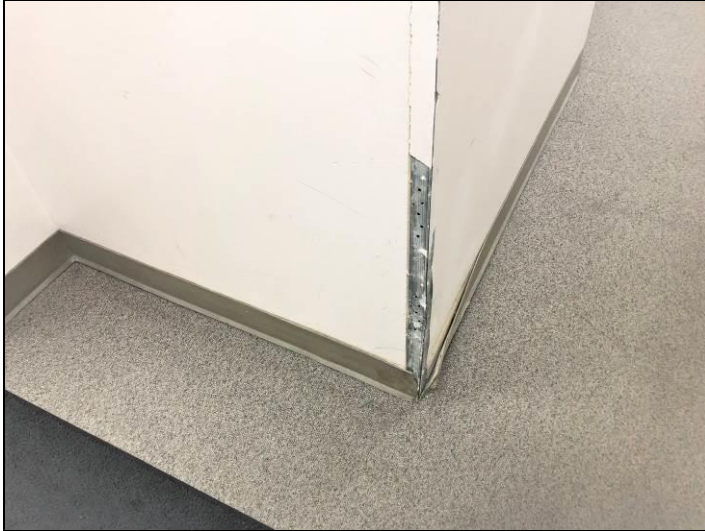
10. View of the drywall (sheetrock) and joint compound found on the interior walls located throughout the building. Also shows the non-asbestos vinyl cove base found in various areas within the building.
