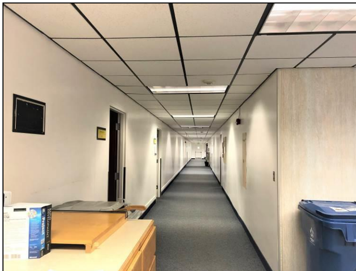
8. View of the non-asbestos 2'x2' ceiling tiles found in various locations throughout the building. Also shows the non-asbestos vinyl wall covering found on the hallway walls.
