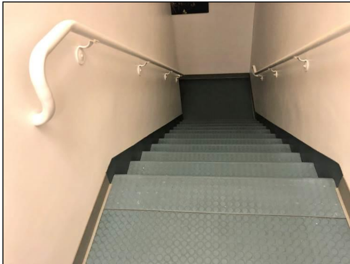
17. View of the non-asbestos blue raised dot vinyl flooring found within the stairwells. Non-asbestos 9-inch vinyl floor tiles were found beneath the vinyl flooring.
