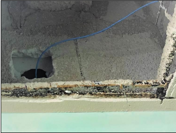
4. View of the non-asbestos CMU block/mortar and the stucco-like plaster finish found on the ceilings and walls found in various locations throughout the building.
