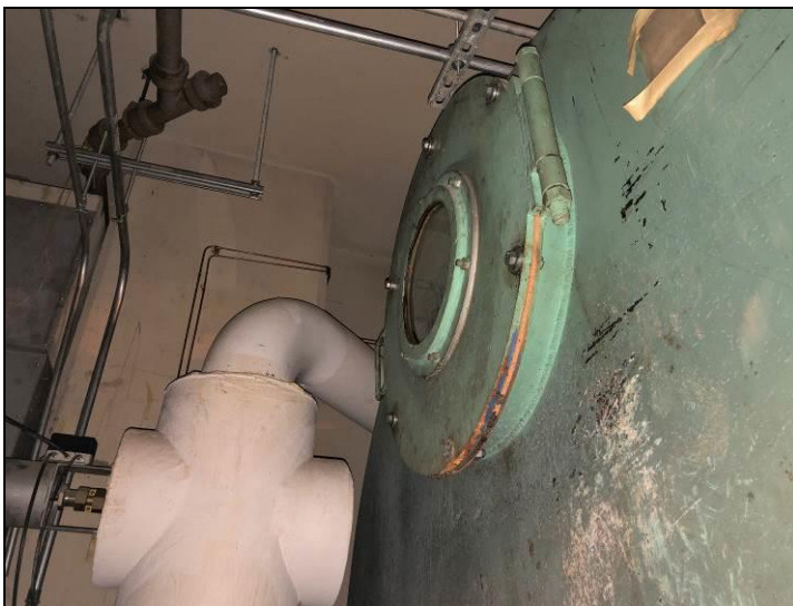
18. View of the non-asbestos gasket material located at the inspection plate found on the north end of the lager tank located in the basement mechanical room.
