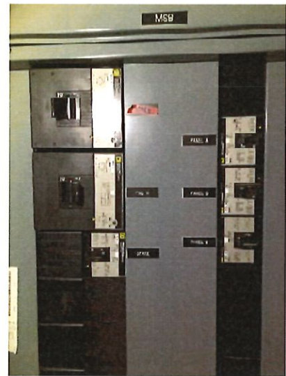
MSB LOAD BREAKERS
