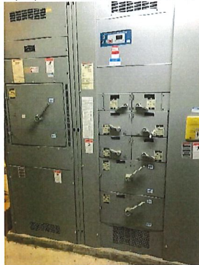
The Existing Main Switchboard
