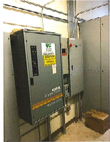
The Existing ATS
