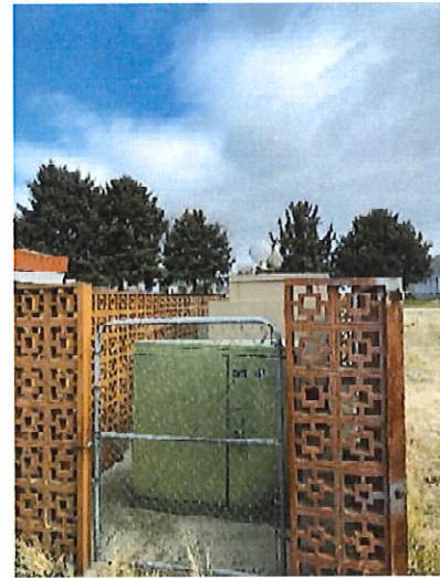
TRANSFORMER AND GENERATOR
